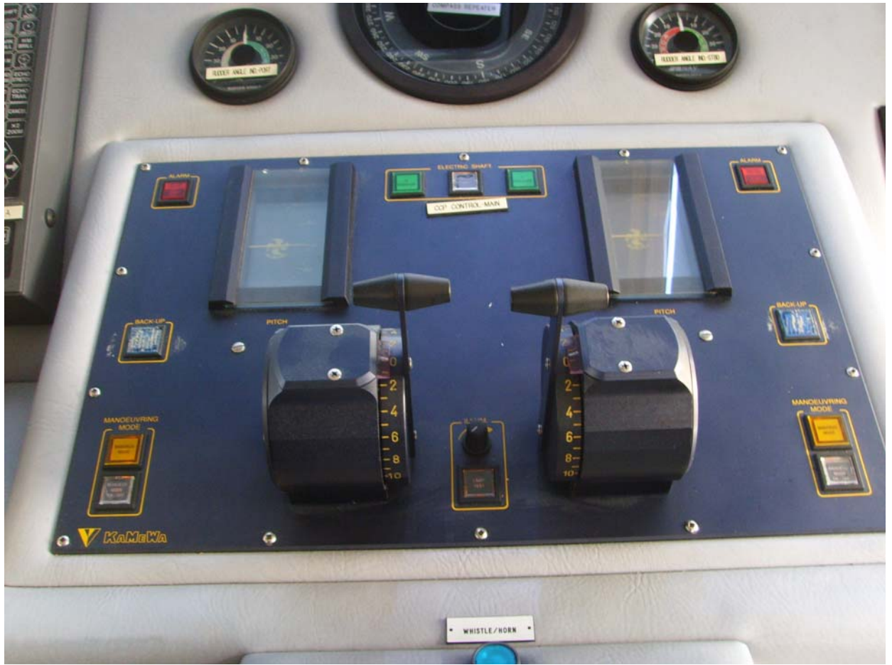
Combinator Control Panel
